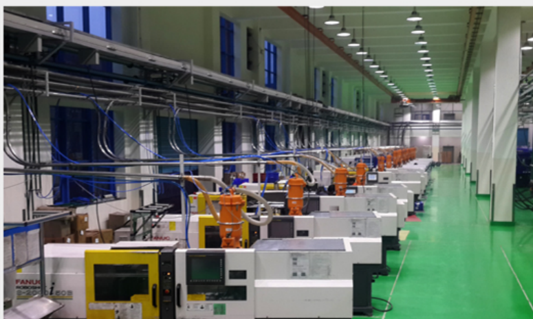
Central Conveying System for 34 Injection Moulding machines with flexibility of using any material on any machine.
