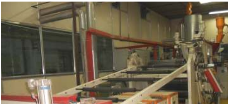
Drying and Crystallizer with PET recycling plant
