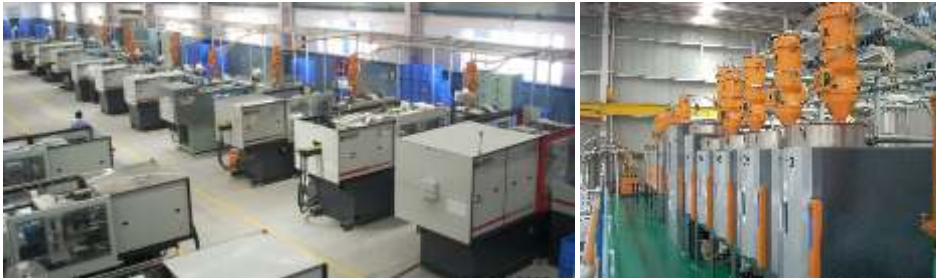
Central Dehumidified Air Dryer and material conveying system for automotive components
