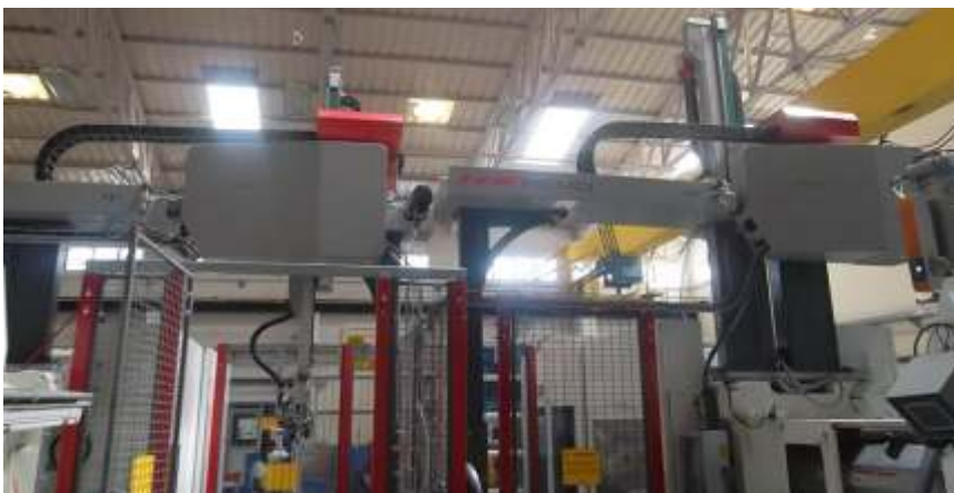
Three axis servo robots installed between two all electric Injection Moulding machines for automotive product moulded with two different polymers
