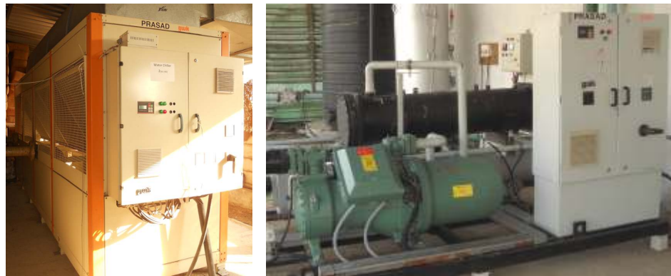
Screw Chiller - Air Cooled and Water Cooled installed with PVC and PE pipe plants
