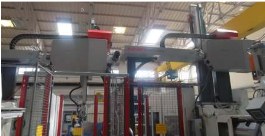
Three axis servo robots installed between two all electric Injection Moulding machines for automotive product moulded with two different polymers
